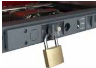
“Disconnected” position locking by padlock.
